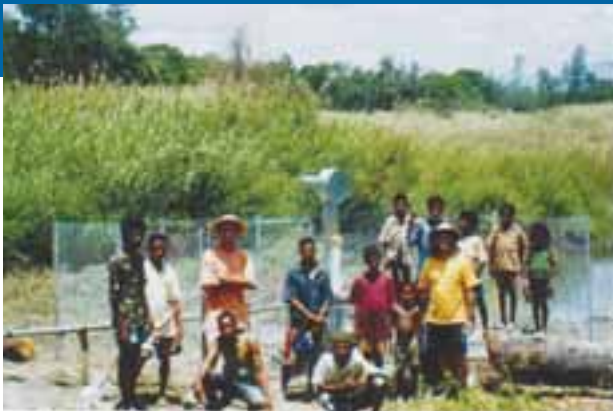
Sun Mill installation Manatuto, East Timor
