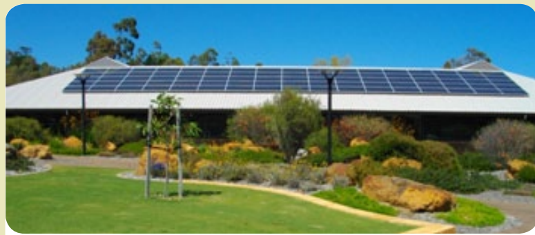
Solar array on administration building
